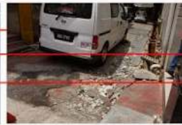
Issue: Poor road condition may cause road accident.
