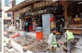
Issue: Construction in progress cause jam and sound pollution.
